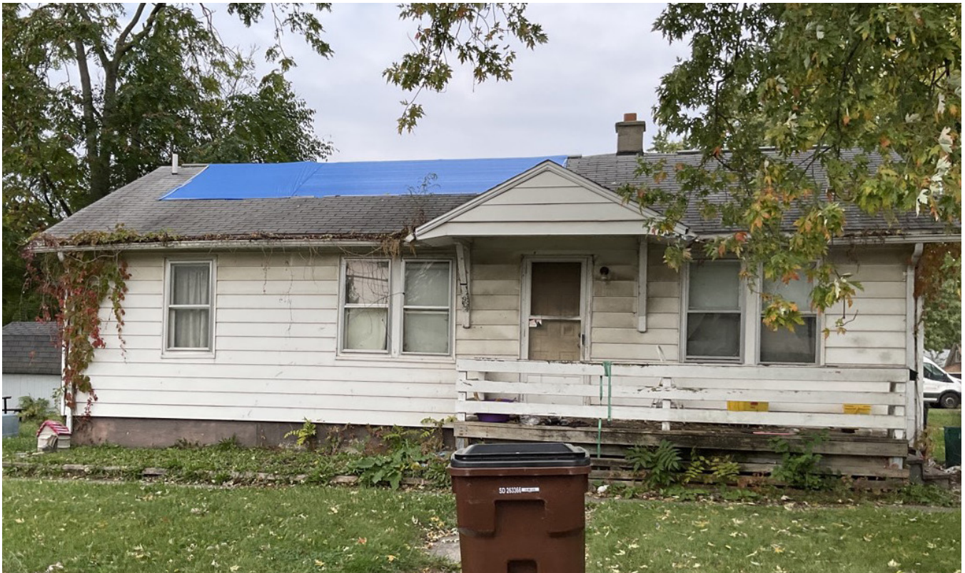
Hole in roof, vegetation in gutters, and porch quality require repair and maintenance.
